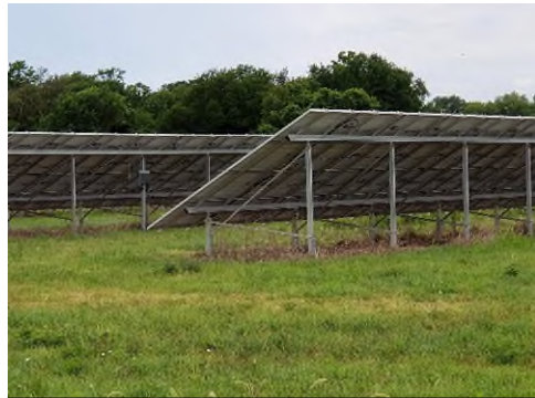
Example of a Solar Conversion System, Ground-mounted
