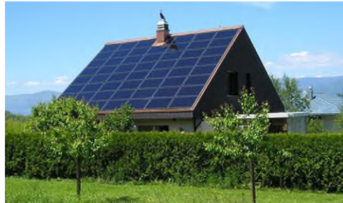
Example of a, Structure-mounted Solar System
